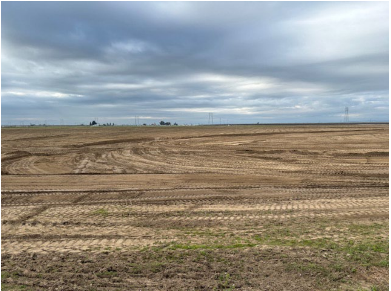
Over-Excavation beneath Levee Embankment between Basin 2 and Basin 3
