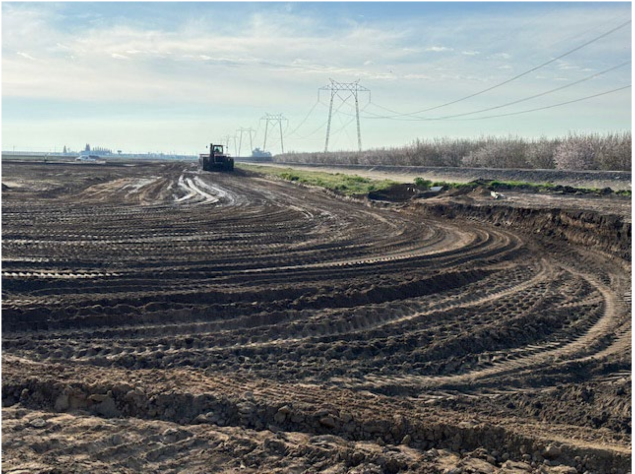
Filling and Compacting on Keyway and Levee in Northwest Corner of Basin 4
