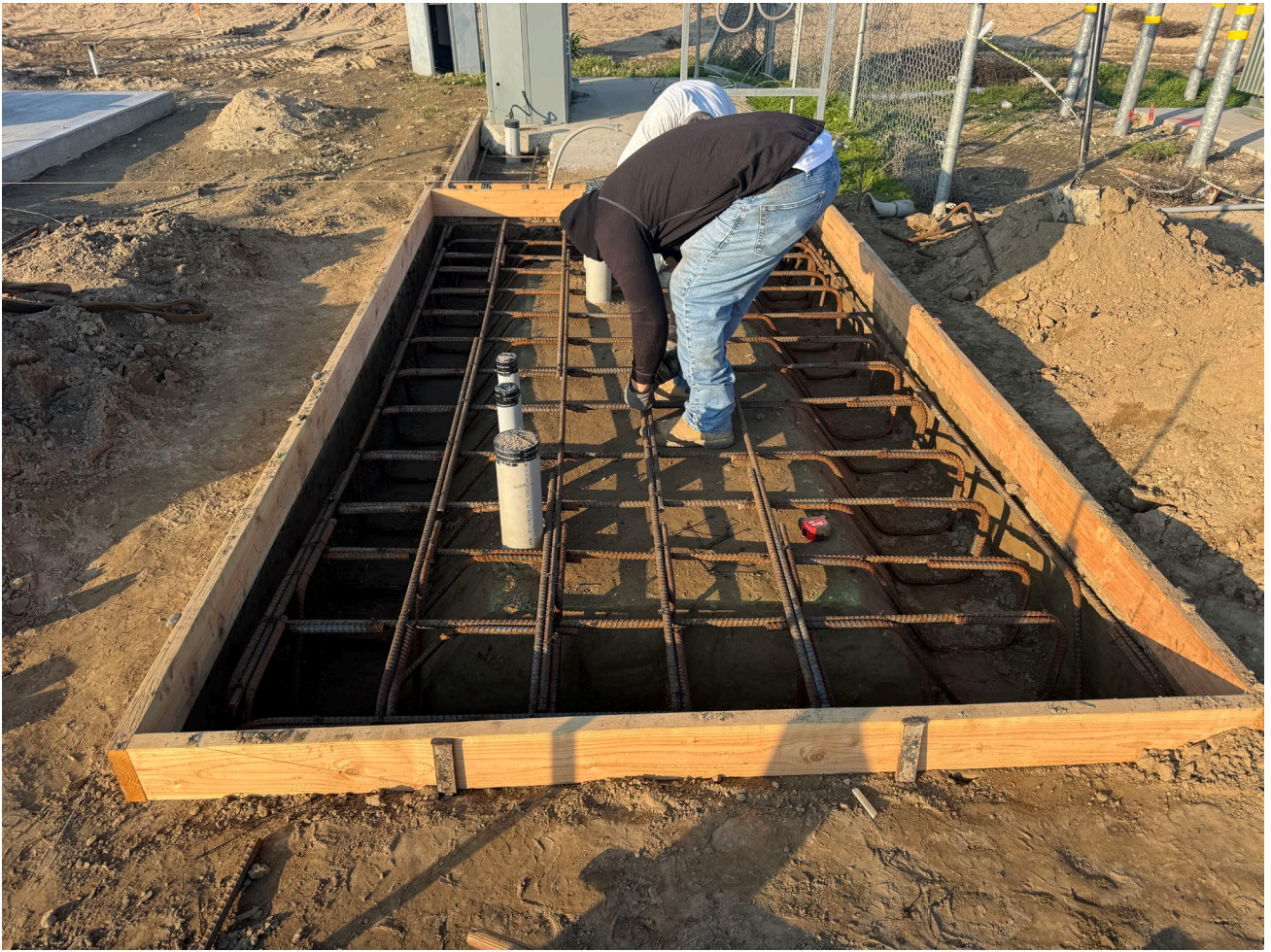
MCC Pad at WE-AG
