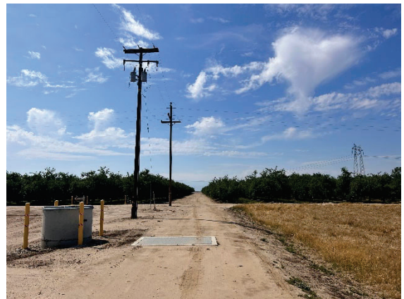
Photo #12 View of the adjacent pole-mounted transformers and ag water infrastructure, facing south.
