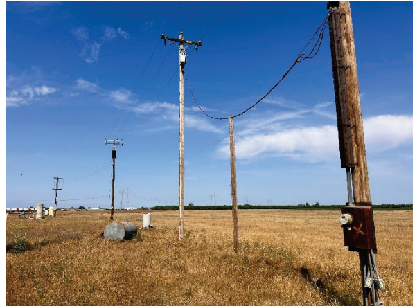
Photo #8 View of the two pole-mounted transformers on Site in the northeastern corner, facing northwest.
