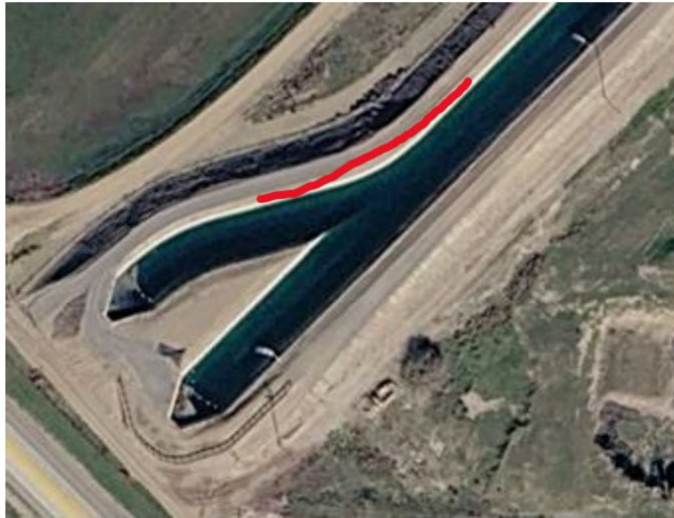
Figure 3. PP1 afterbay after I5 siphon needs to have a wider smoother transition to the main pool.
