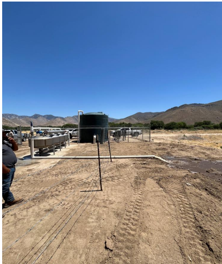
Figure 2 Onyx Water Treatment Performing Backflush Cycle
